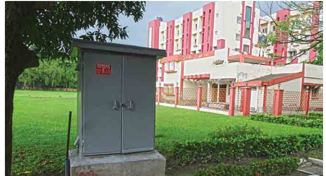
Refabricated Feeder Pillar
