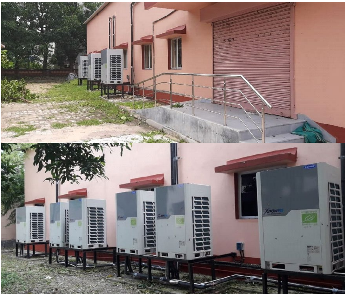
Lab-1 VRF Air Conditioning Machines
