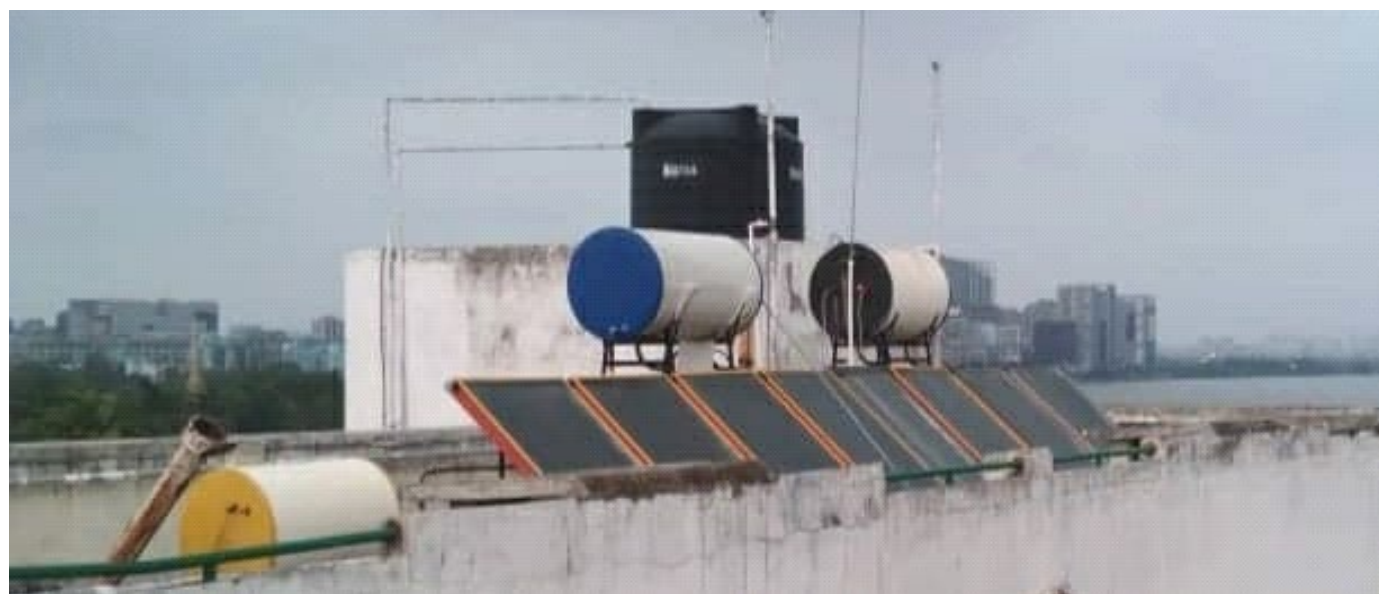
Additional 2 Nos. 500 LPD Capacities Solar Water Heating System
