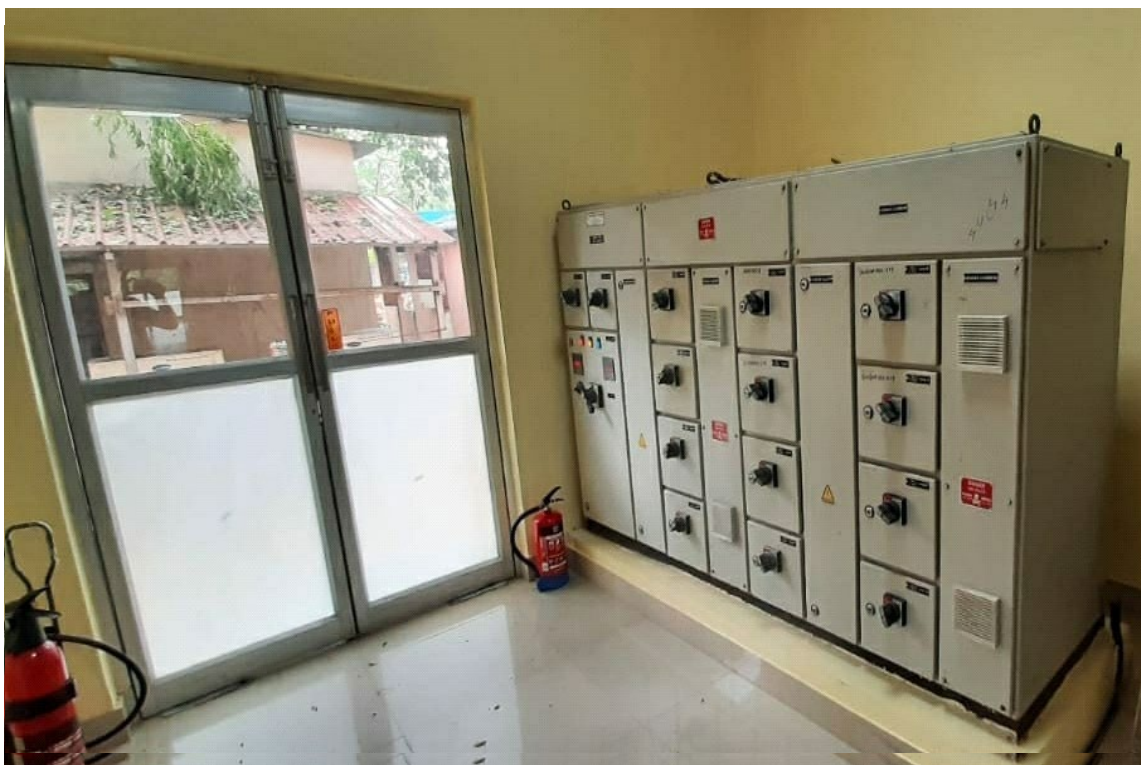
Lab-1 Main Electrical Panel
