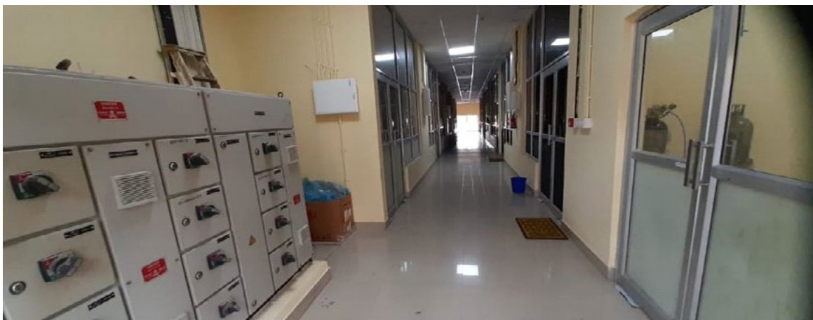
Lab-2 Main Electrical Panel
