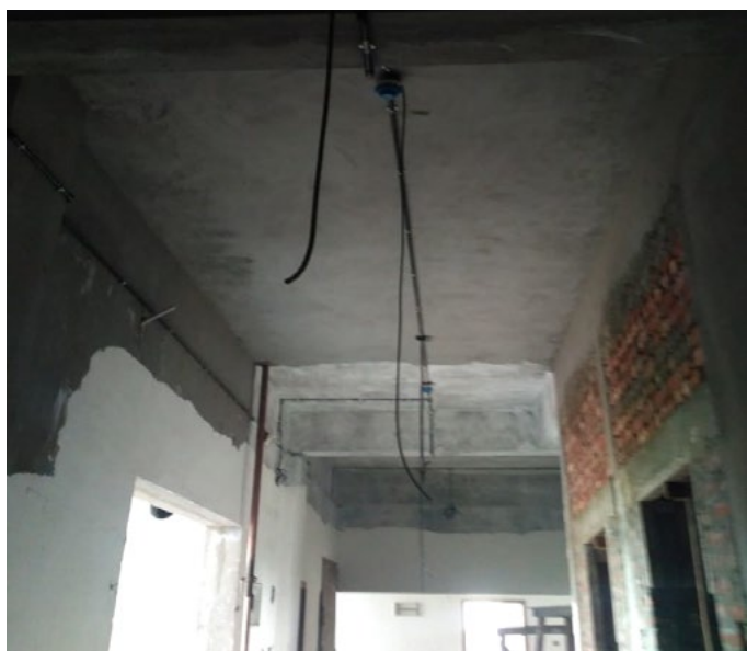
Fire Detection System
