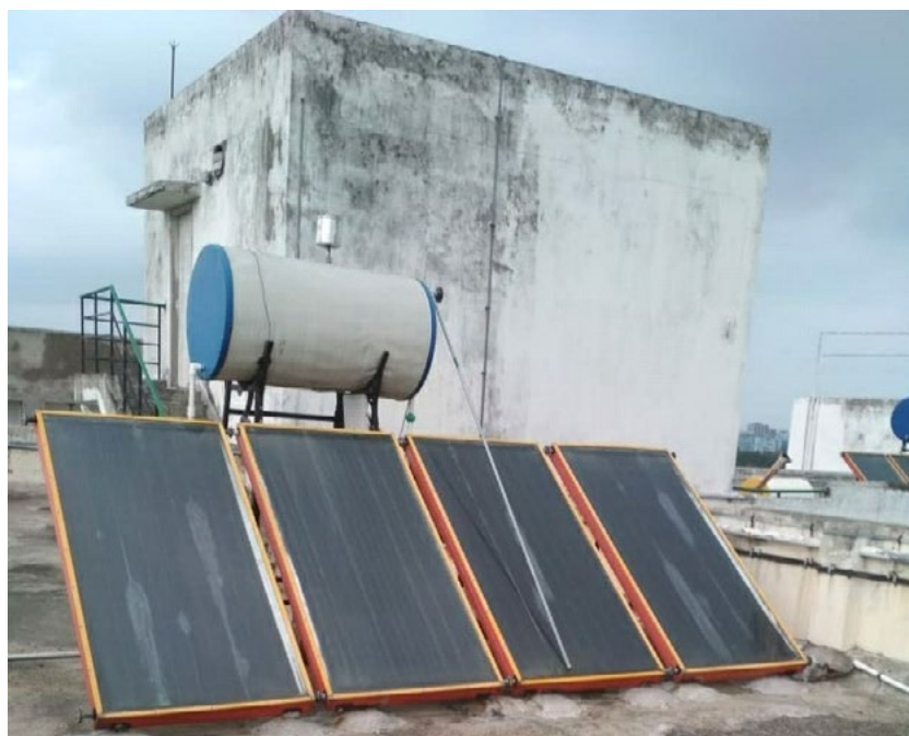
Another 500 LPD Capacity Solar Water Heating System
